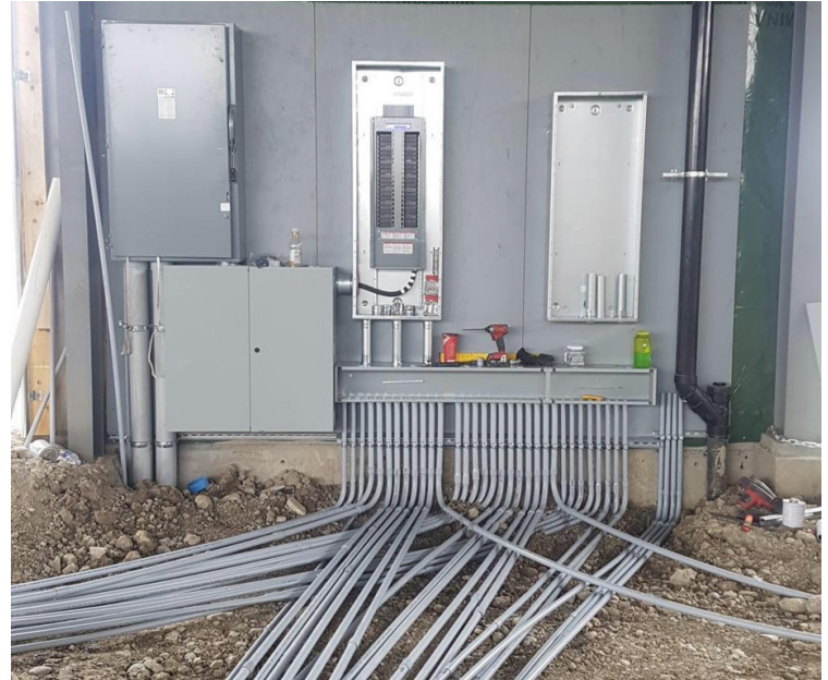
PVC 90's? Aren't you concerned about your jet line/rope cutting through them when you pull the wires? We always use rigid 90's underground.
